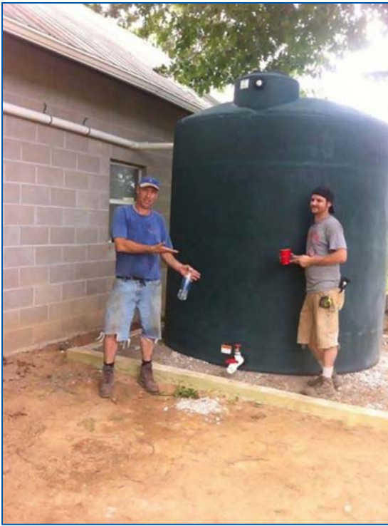
Newly installed cistern attached to farm building. Photo: Guy K. Ames, NCAT
